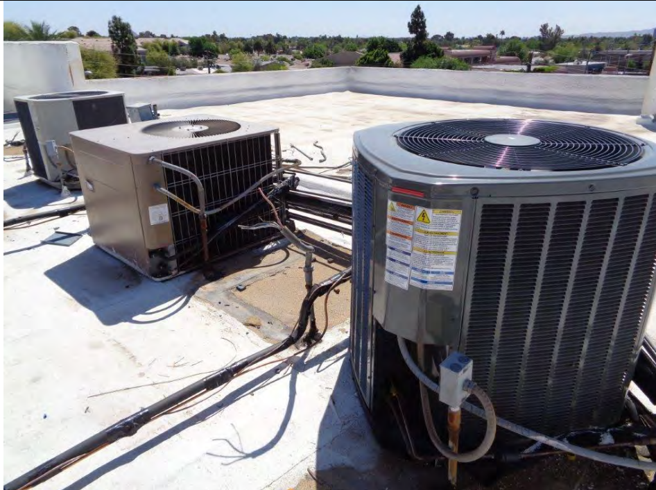
Typical electric rooftop HVAC units
