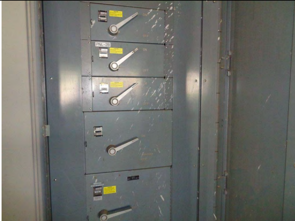
Main electrical panel
