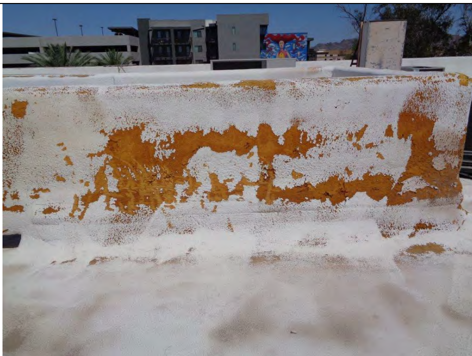
Typical foam degradation
