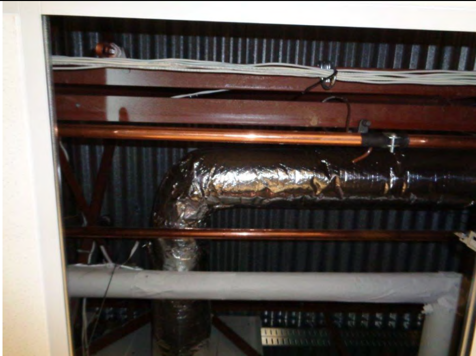
Copper water distribution piping
