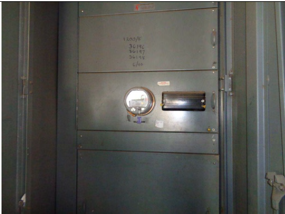
Main distribution panel
