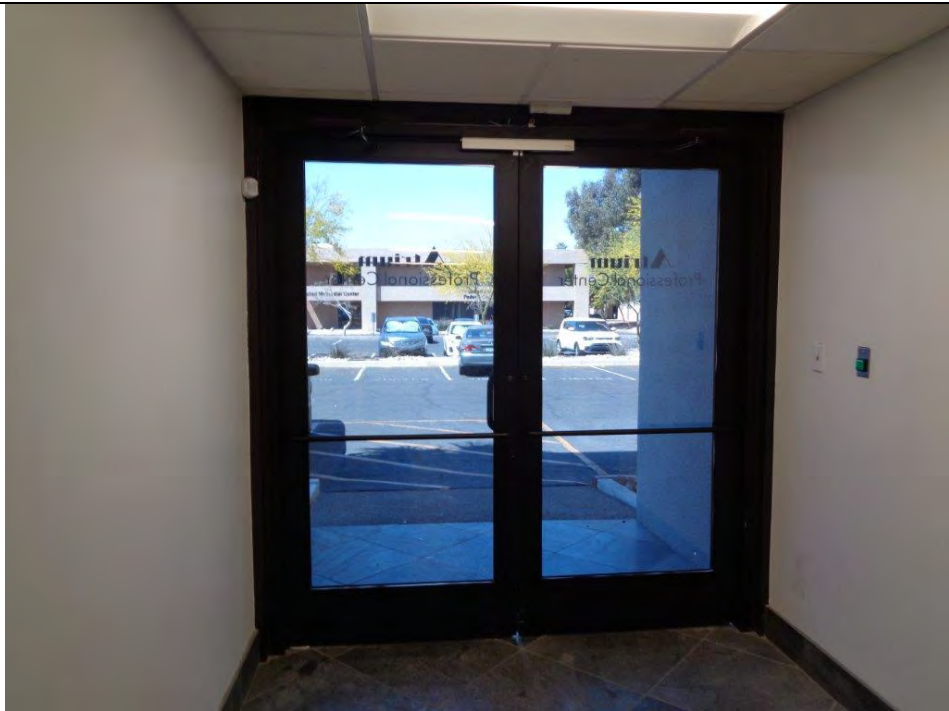
Tenant entry doors with key card access
