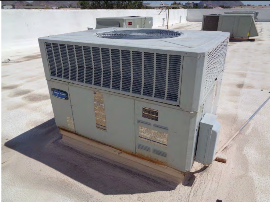
Older RTU from 2010
