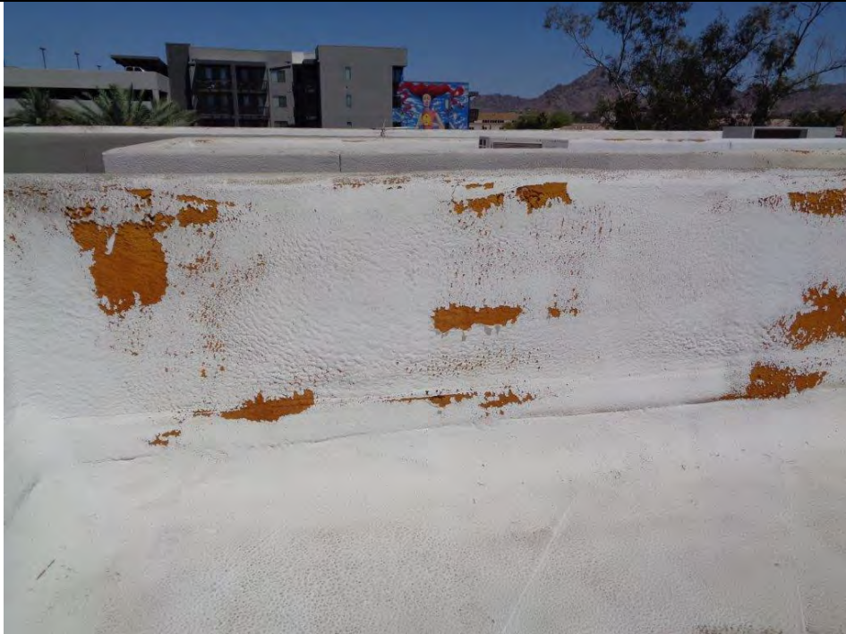
Typical foam degradation and delamination
