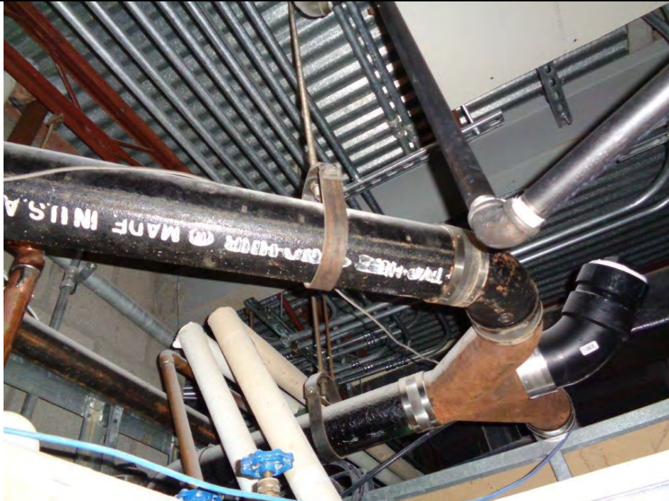
Cast iron waste piping
