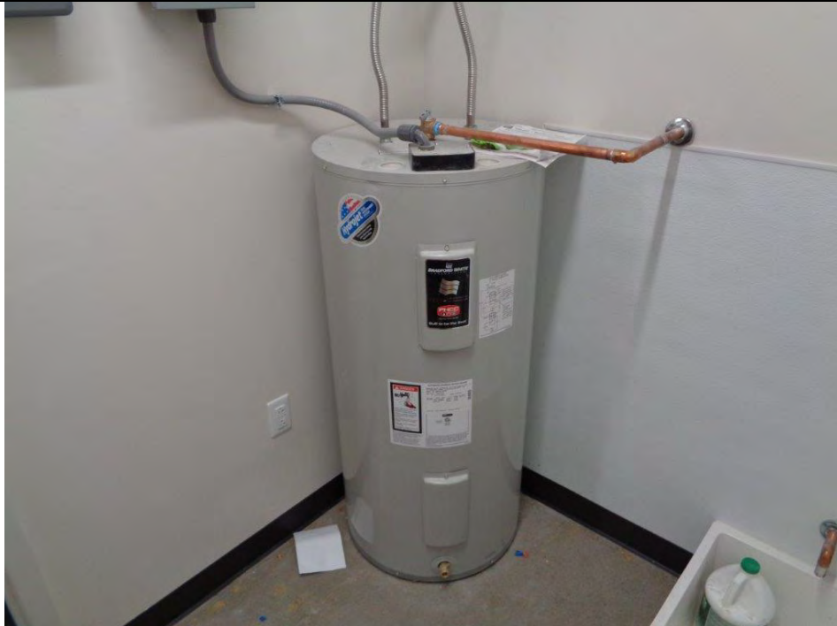
Hot water heater
